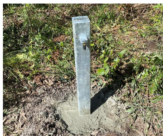
Installed groundwater monitoring well with steel monument.
